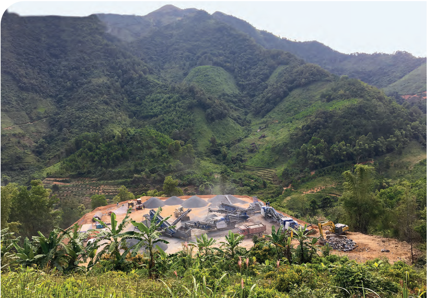
The Licogi 16 team worked with Kleemann plants in a quarry 40 km south of Lang Son.
